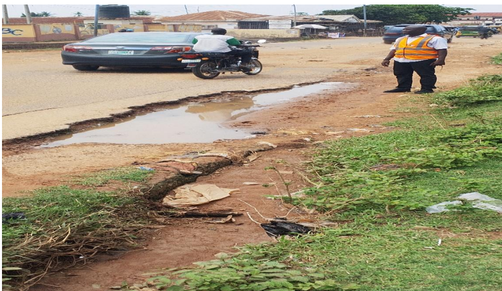
Figure 2. Surface water accumulation and drainage-related pavement distress.
